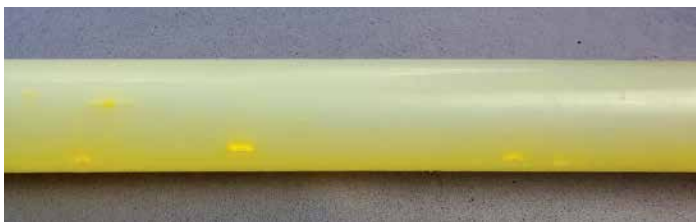
Chlorine induced cracks in PEX piping.
